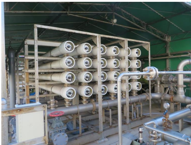
RO造水設備(ナイカイ塩業内)
